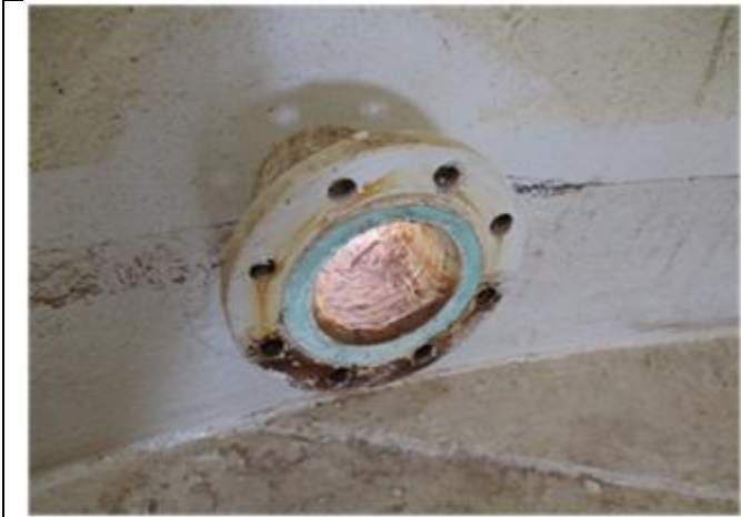
Water Drain Off (Internal) - Size: 4 inch.
